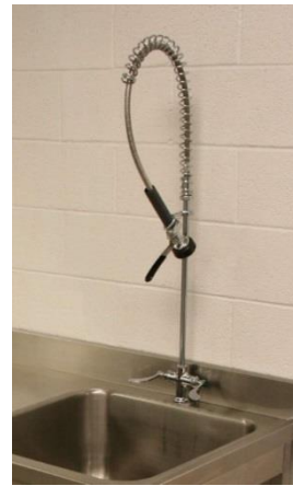
Hot and cold spray rinse
